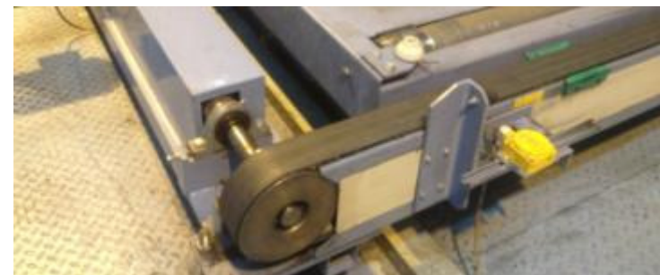
Old conveyor set-up
